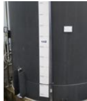
Water tank 10,000 litre capacity Lot 62
